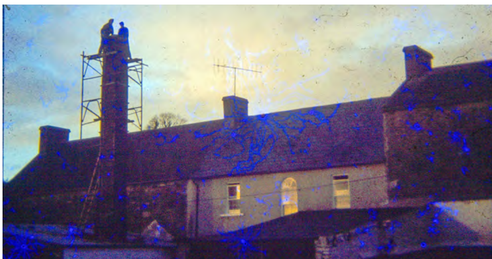
Photo from the early 1970s showing the removal of the chimney stack from Timoleague creamery. It is taken from the bottom of the creamery yard, the building on the right is the Courthouse, then Harringtons and the creamery itself. On the scaffolding are the late Tommy O'Rourke and Steve O'Mahony. Photo courtesy of Gearóid Holland
