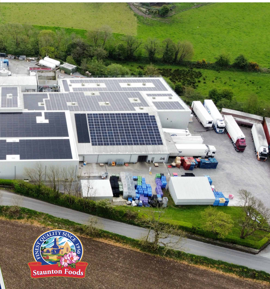
Staunton Foods roof-top solar installation.
